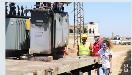
Syria. The ICRC rehabilitates an electrical power network and water-pumping station. See more here .
