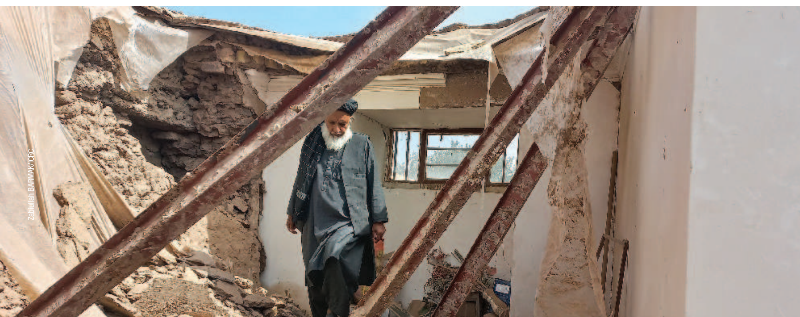
A man inspects his home, which was damaged during the earthquake in Herat's Zenda Jan area.
